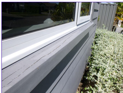
Recommend painting sill
