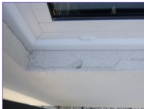
Recommend repairs to sills
